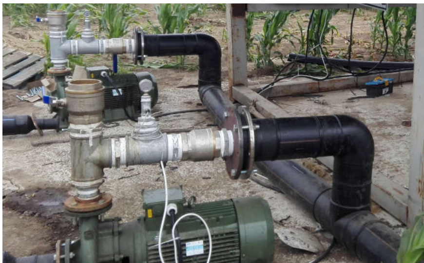
NR. 2 IR 50-250ND with control panel with inverter BULGARIA IRRIGATION IN A CORN FIELD
