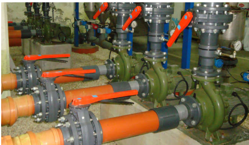
NR. 25 IR4P 65-250NB SPAIN PVC PRODUCTION PLANT
